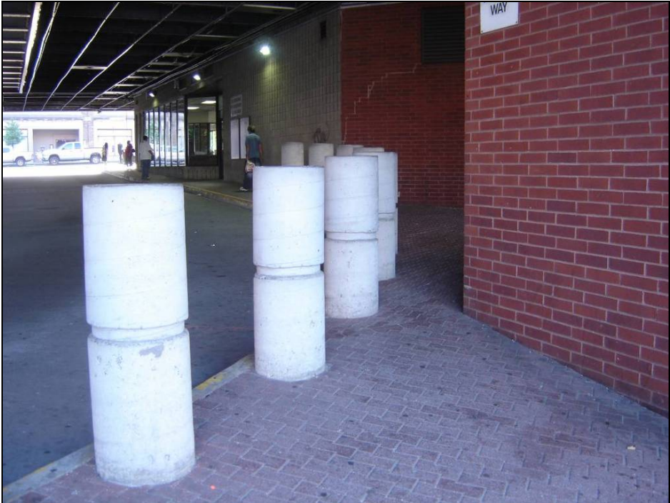
Figure: These bollards obstruct wheelchair passage from Pleasant Street to the bus bays and waiting area. Wheelchair passengers must continue around the block and through three doorways.
